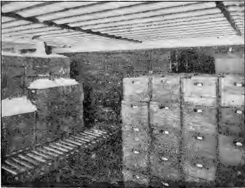
FIG. 10.—Milk-storage room using direct system of cooling with cooling coils overhead. Note iron plates in floor.
